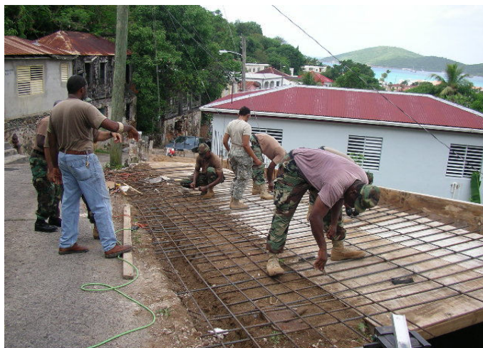
Volunteers from the V.I. National Guard work on the parking slab of Habitat-VI's first home at Adele Gade.
